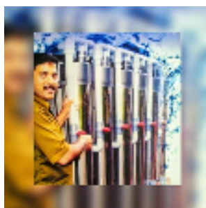
RICHU'S WATER FILTER JACHAR HOSPITAL, KERALAM 25,5000Ltr /day WATER TREATMENT PLANT INSTALLED IN 2018/2019
